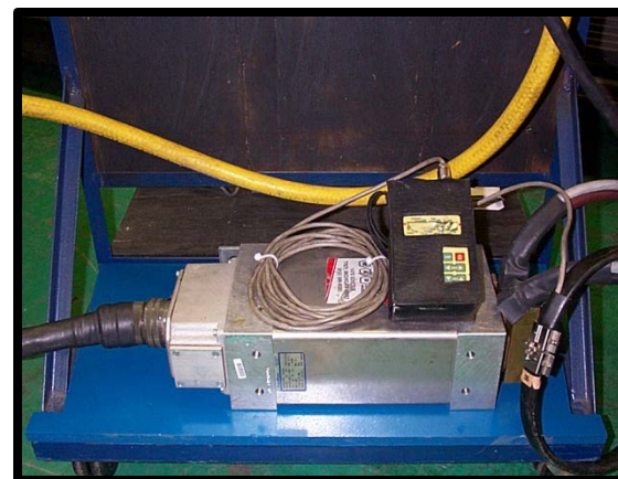
60KVA Weld Transformer
